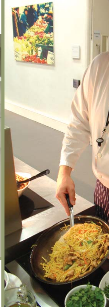
Centrepiece of the main kitchen is a large central island suite fitted with equipment including high pressure steamer, bratt pans and tilting kettle. Backing this up are combination ovens and ranges.
